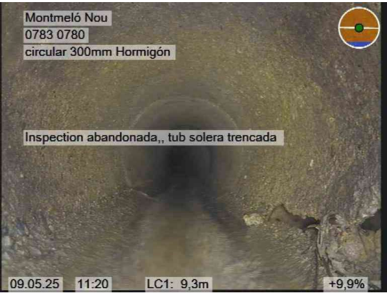
9, 00:05:43, 9.30m Inspection abandonada,, tub solera trencada
