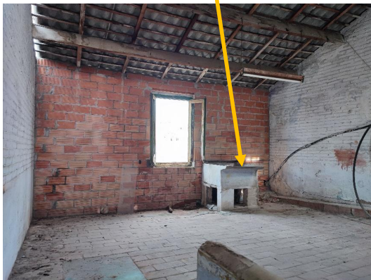
Safareig Contingut amiant
