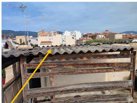
Cobert Contingut amiant – 6 m2
