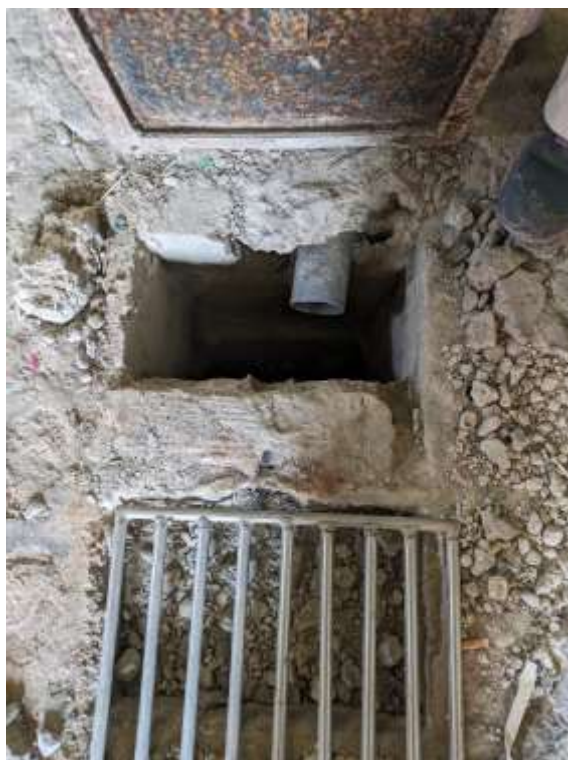
Embornal interior existent
