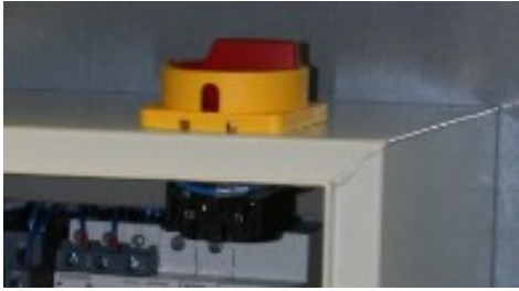
Picture 13: Main switch on top of control box
