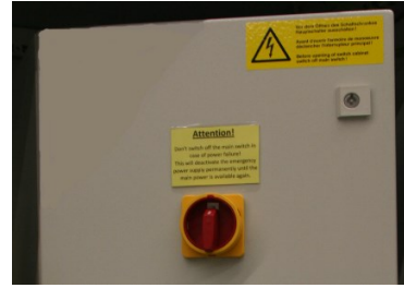
Picture 14: Main switch on in control box door
