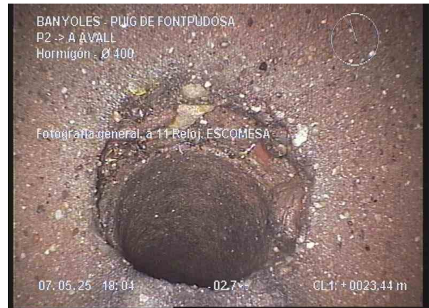
P2-A AVALL_bb682e0c-2a4e-408f-a80e-a9f3d18d82d2_20250507_181414_443.jpg, 00:02:47, 23.40m
