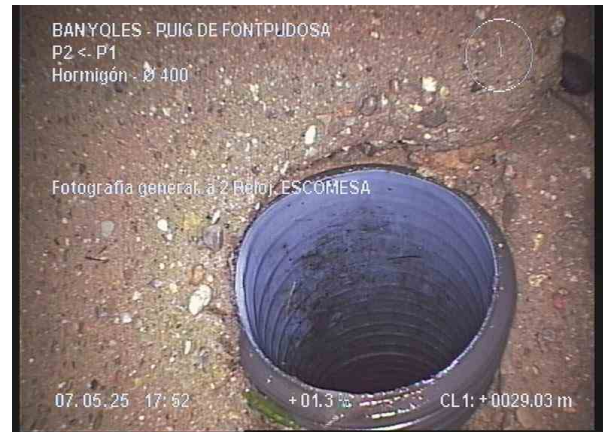
P2-P1_ea6cbf8f-961e-475a-a3f2-d8df27b9d4b6_20250507_180214_390.jpg, 00:03:14, 29.00m Fotografía general, a 2 Reloj
