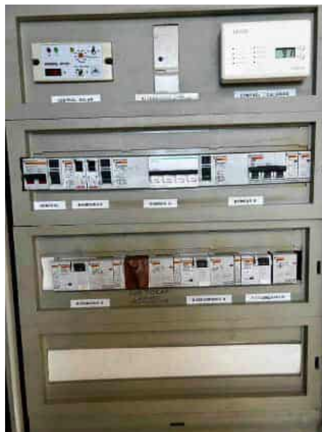
Foto 5: Bombes circuit primari ACS solar no operatives
