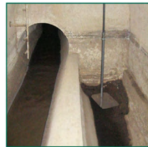
FLOW MEASUREMENT IN NARROW UNDERGROUND U-SHAPED CHANNEL
