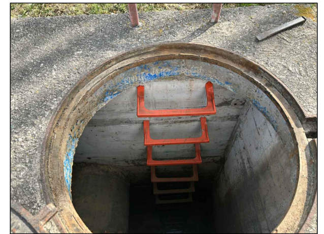
Interior arqueta G5-2D
