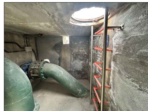
Interior arqueta B2-68
