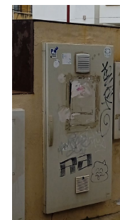
Fig 10: Armari exterior FTTH
