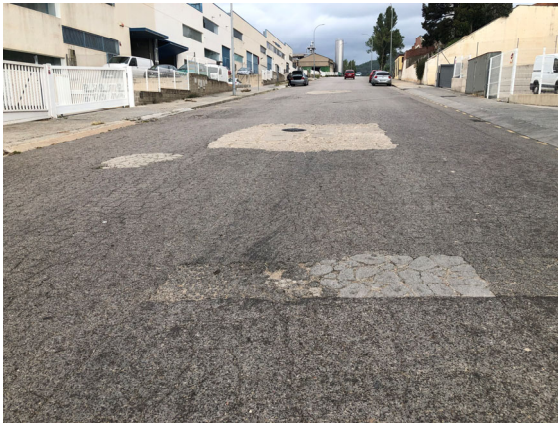
Rases mal executades
