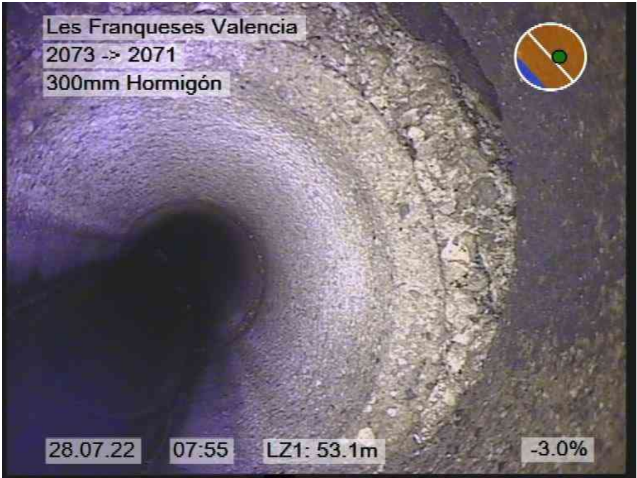
62.jpg, 00:09:43, 53.10m OBSERVACION GENERAL
