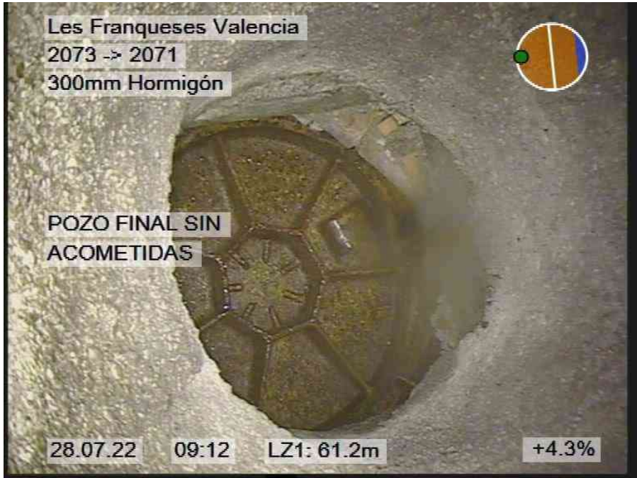
68.jpg, 00:12:56, 61.20m POZO FINAL SIN ACOMETIDAS
