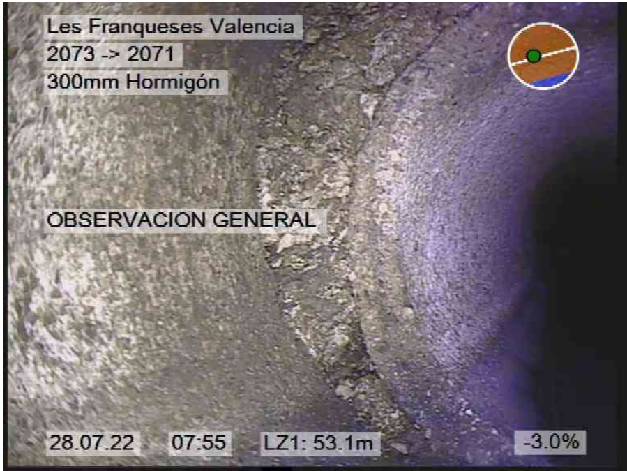
61.jpg, 00:09:43, 53.10m OBSERVACION GENERAL
