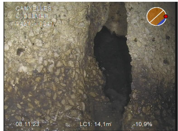
P401-P241_1297fada-1c43-4971-9129-0d68b2db346d_20231108_093055_968.jpg, 00:07:15, 14.10m Observación general / JUNTA ROTA
