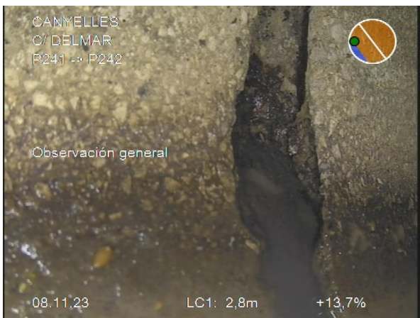
P242-P241_3acf07c0-5a60-4d22-97fe-a03f49f6fbff_20231108_101037_338.jpg, 00:01:14, 2.80m Observación general / JUNTA ROTA
