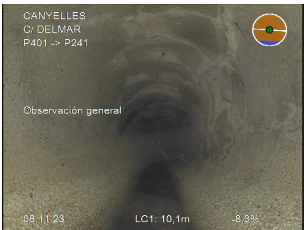
P401-P241_005fa638-c59d-423b-a4d2-c3d58be0cd67_2023108_092733_372.jpg, 00:04:33, 10.10m Observación general / FISURAS GENERALES
