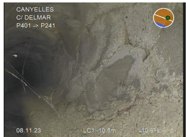
P401-P241_9632c553-441e-4536-a558-476fb75a87d3_2023108_092741_834.jpg, 00:04:33, 10.10m Observación general / FISURAS GENERALES
