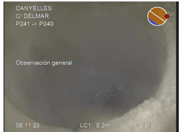
P241-P240_80b44d2d-4e05-4c62-b3c3-42212dde904f_20231108_094307_876.jpg, 00:02:00, 5.20m Observación general / ACOMETIDA DCHO, 2H
