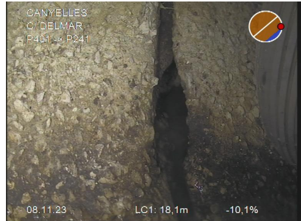
P401-P241_9c3668d5-c9af-4b2d-8635-3d34c06e0d4b_2023108_093538_034.jpg, 00:10:13, 18.10m Observación general / JUNTA ROTA
