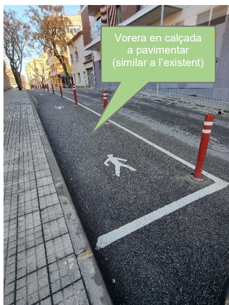
Tram vorera a consolidar
