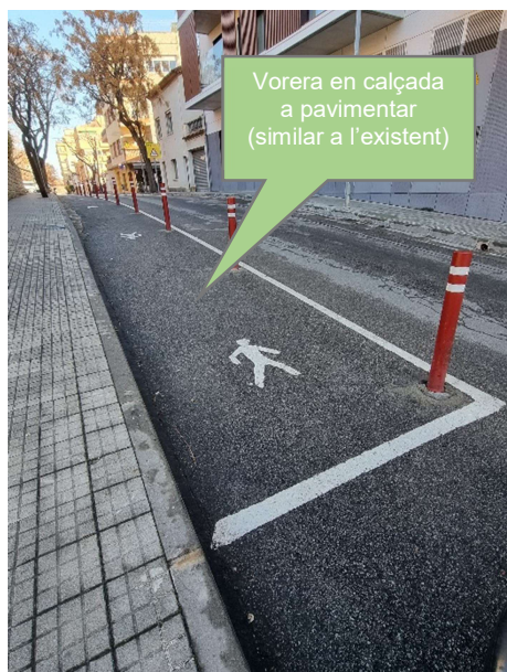
Tram vorera a consolidar
