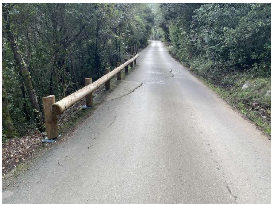
Manca abatiment lateral
