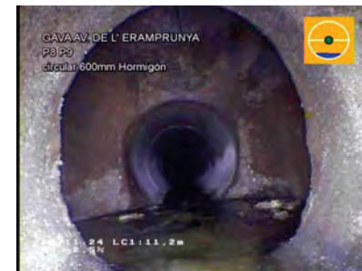
P8 A P9_b2cce555-9497-4492-bbde-d56d64bf7884_20241129_090 658_542.jpg, 00:01:39, 11.20m Nudo de final, registro., P9
