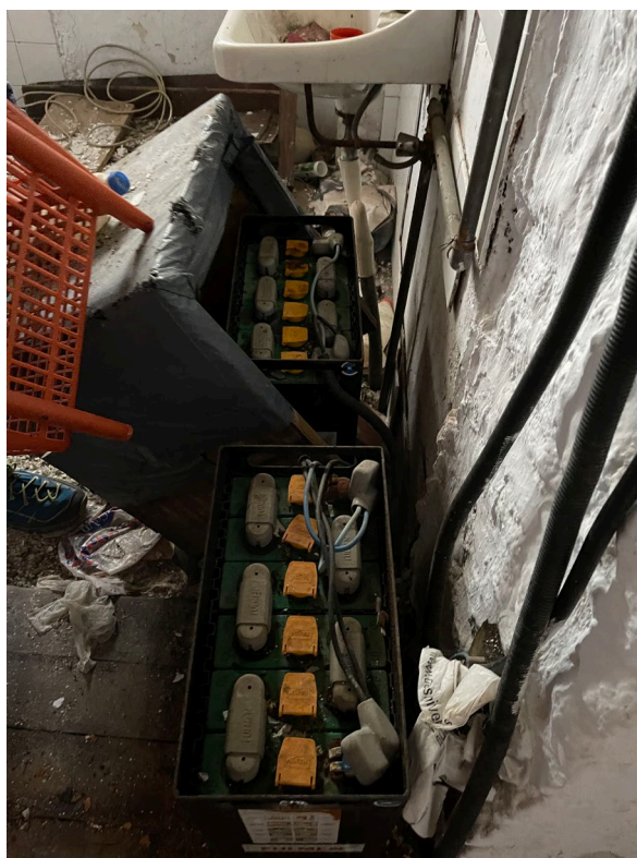
Presencia de residus contaminants, bateries.
