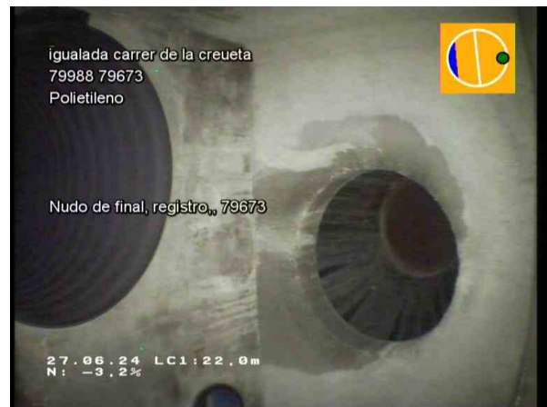
29764_bdf03654-9cf4-42b1-8e6e-5e705e89b85f_20240627_102130_923.jpg, 00:03:21, 22.00m Nudo de final, registro,, 79673
