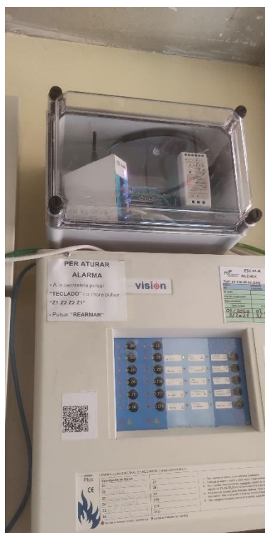
Foto 4: Armari Router IXON a Consergeria
