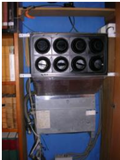
053 Fan-coils Sala de Reserva
