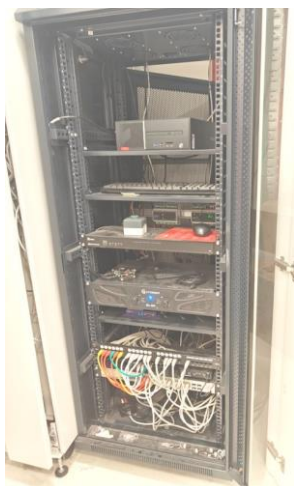
Armari rack elements centrals
