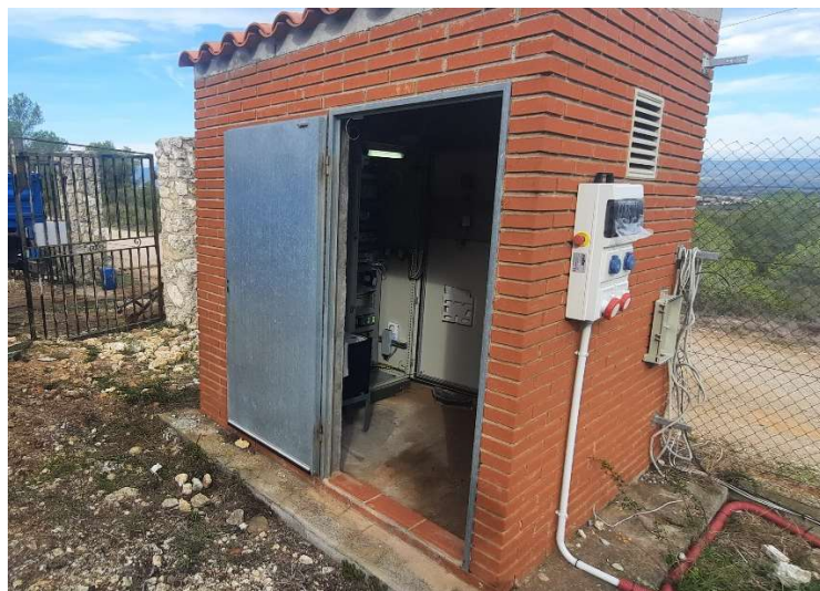
Armari electric i caseta existent
