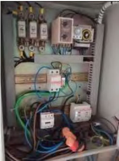
Armari de control interior
