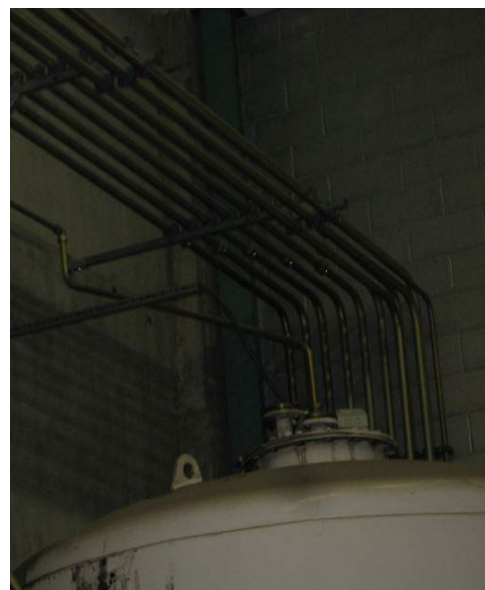
Figura 4. Rack de fluids
