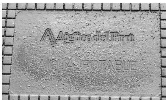
Marcats "Aigua potable"
