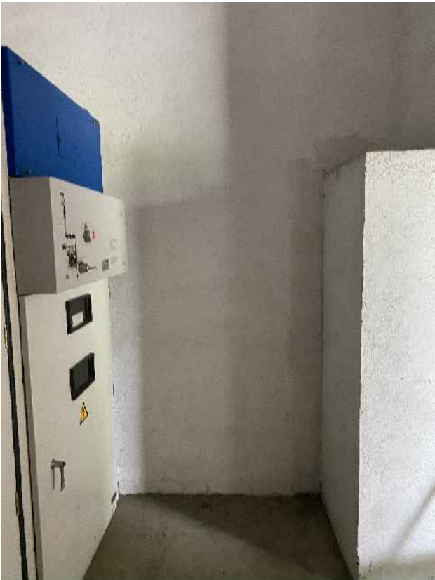
SALA MANOBRA i CABINES A DESMANTELLAR
