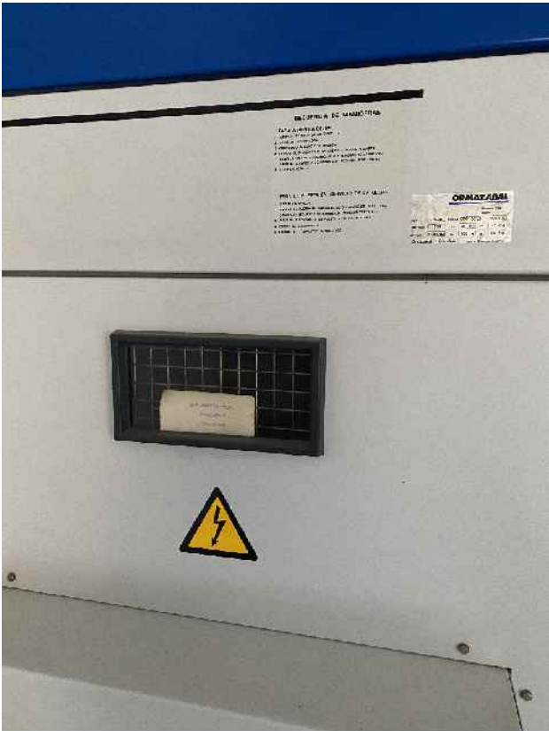
SALA MANOBRA i CABINES A DESMANTELLAR
