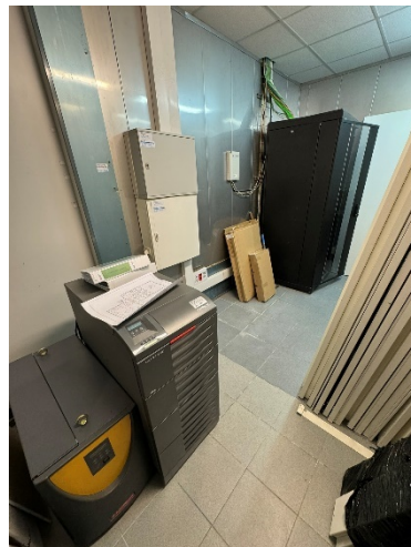
Local Rack i SAI
