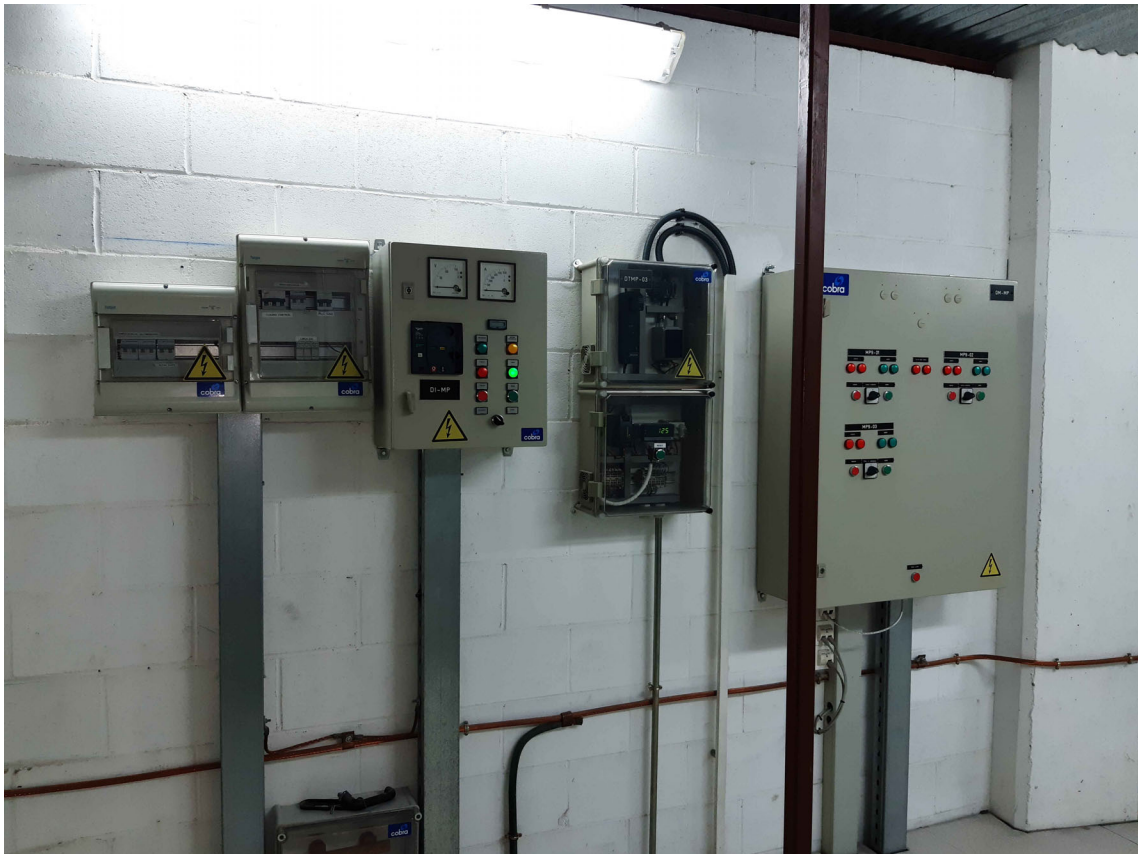
Sala seccionadors Macropou (costat SET SSM)
