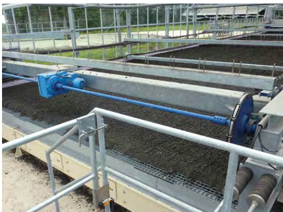
Drive unit at dry sludge area
