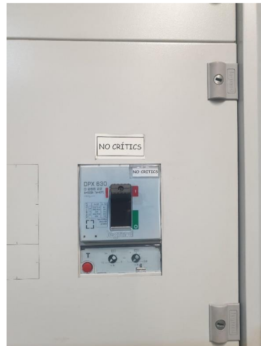
Interruptor general armari no crítics
