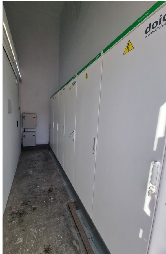
Quadre General BT existent
