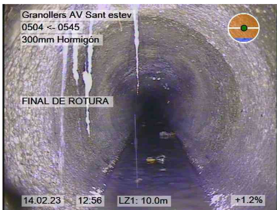
179.jpg, 00:01:42, 10.00m FINAL DE ROTURA
