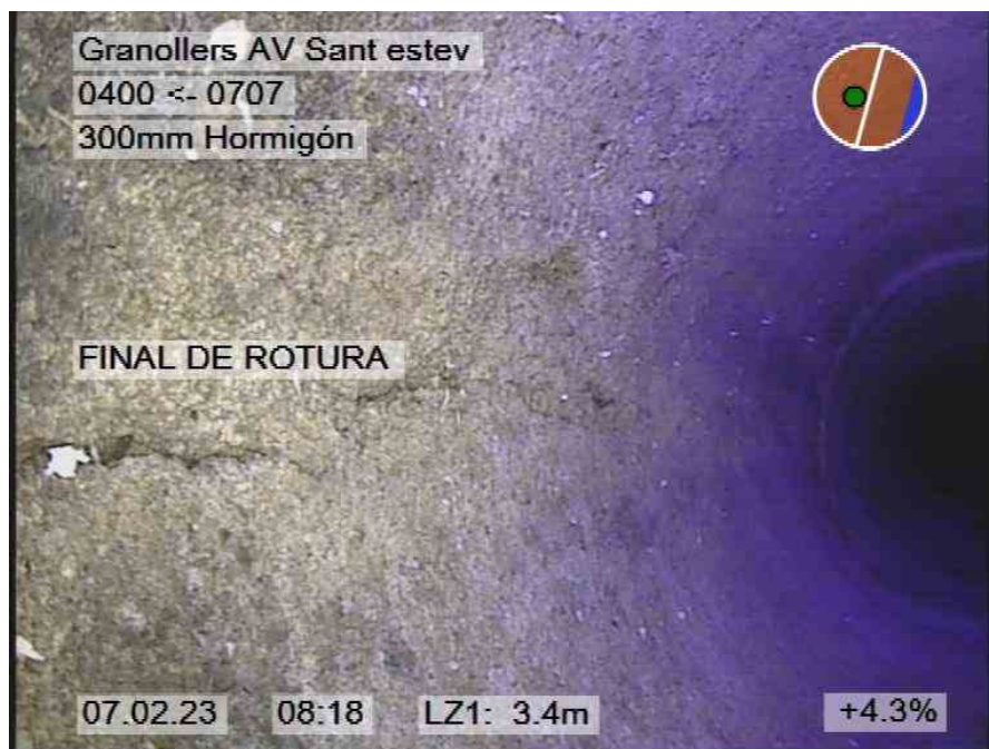
93.jpg, 00:01:04, 3.40m FINAL DE ROTURA
