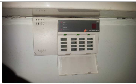
Armari Alarma Foc
