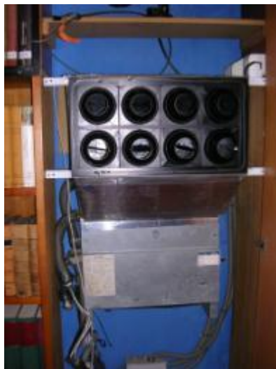
053 Fan-coils Sala de Reserva
